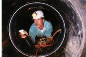
Check for Leaks
