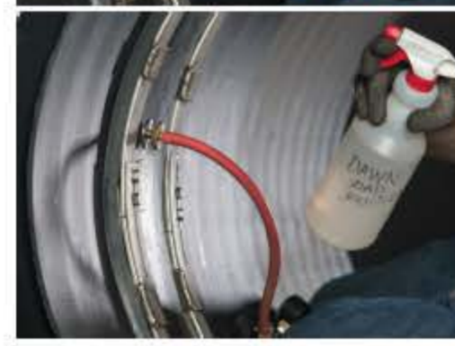
Check for Leaks
